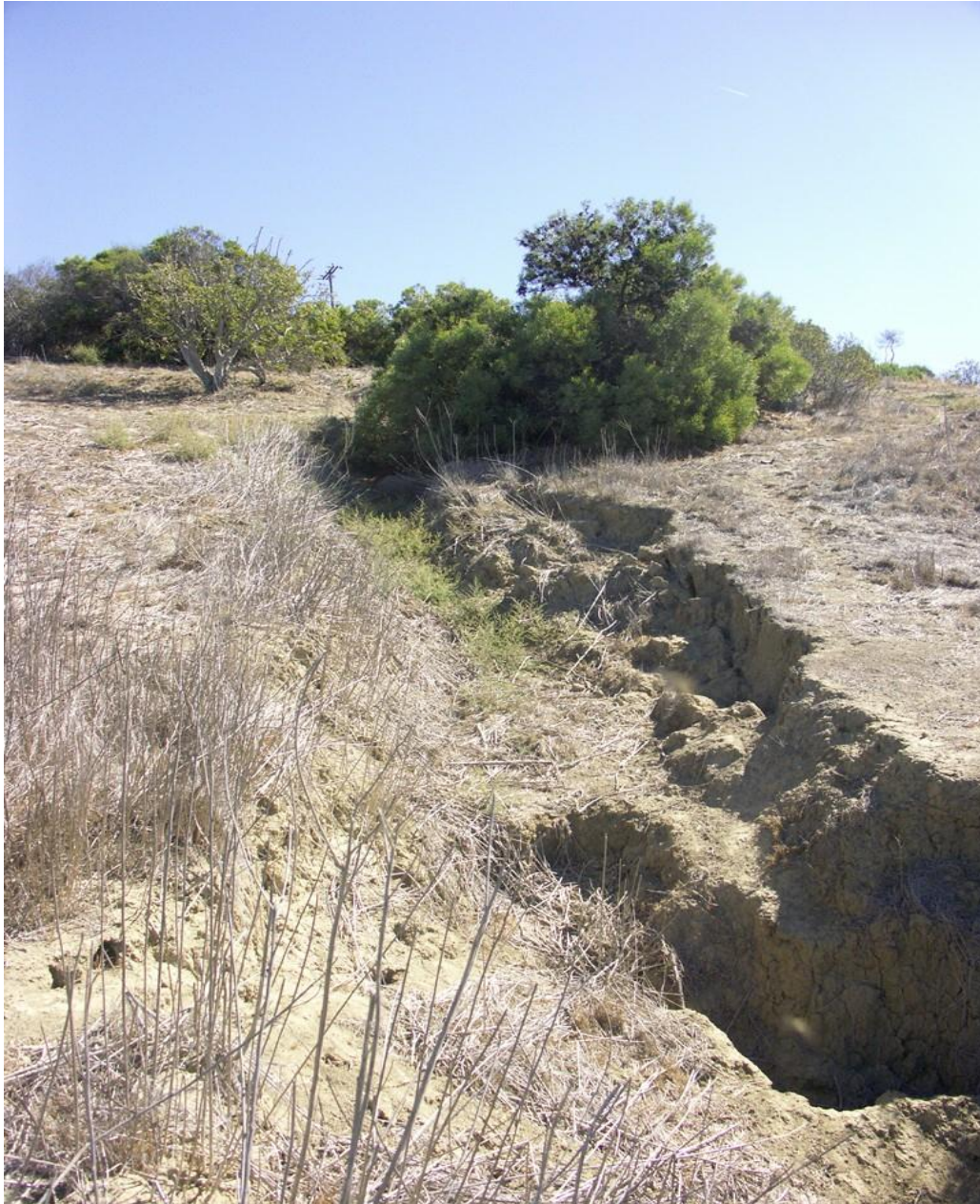
Figure 5. Erosion gully from Runoff Source B and possibly A, that is just above the Lower Parking Lot. It is located along watercourse 8 at 8B.
